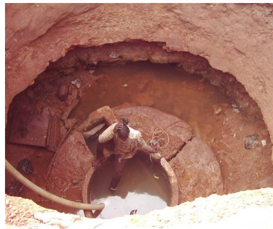
Old abandoned well under reconstruction (note the large diameter of well > 4.5 ft)
